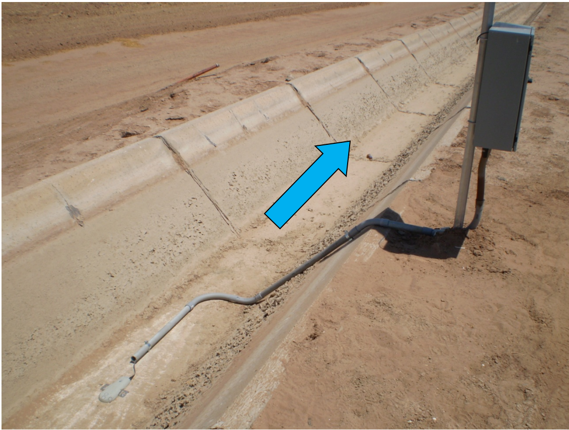
Figure 73. IQ Mounted with Cable Conduit
