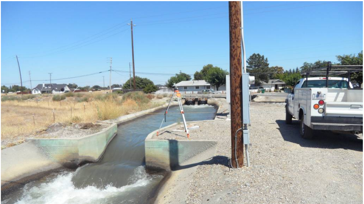
Figure 69. Poor Installtion Site: Control Gate Upstream and Turbulent Flow Downstream
